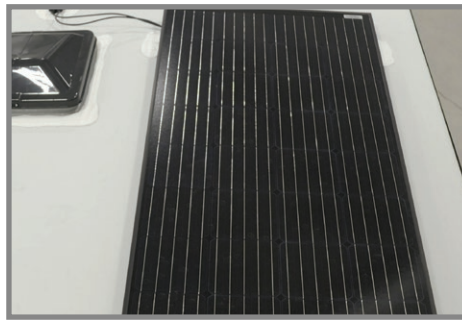
SOLAR PANEL ON ROOF
